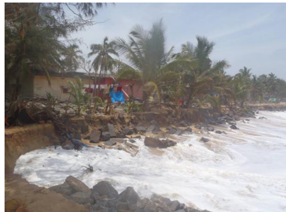
Figure 9. Seawall end erosion at Kasargode
