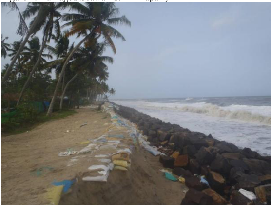
Figure 4. Slumped Seawall at Kattoor
