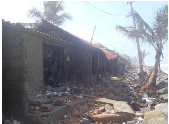
Figure 3. Damaged houses at Valiathura
