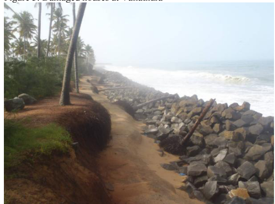
Figure 5. Slumped Seawall at Thanni
